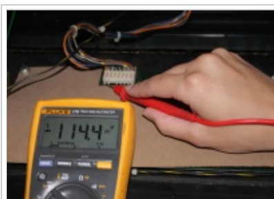
Testing DMD Controller voltages at the display. Note: This picture is a Williams game, but the concept is the same.
